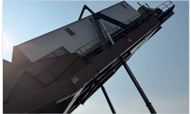
MILL DELIVERY: Hydraulic truck dumper unloading wood chips at the Hibbard Renewable Energy Center in Duluth.
